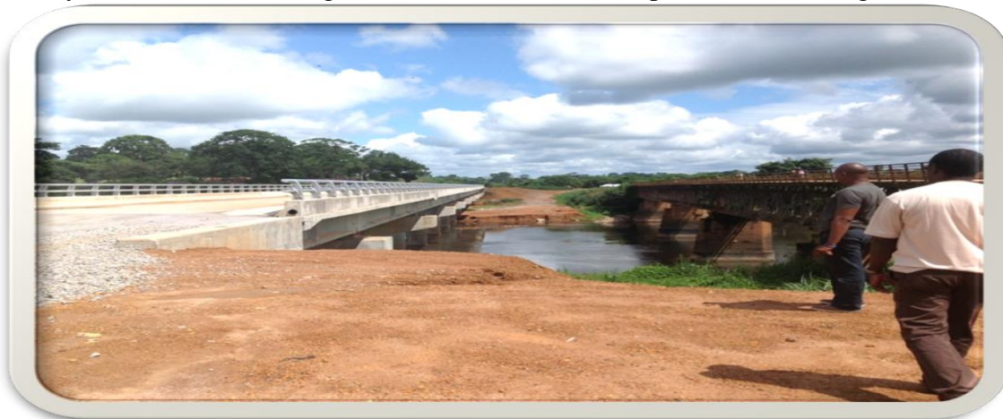
Newly constructed Daru Bridge on the Left and Old one on the right
